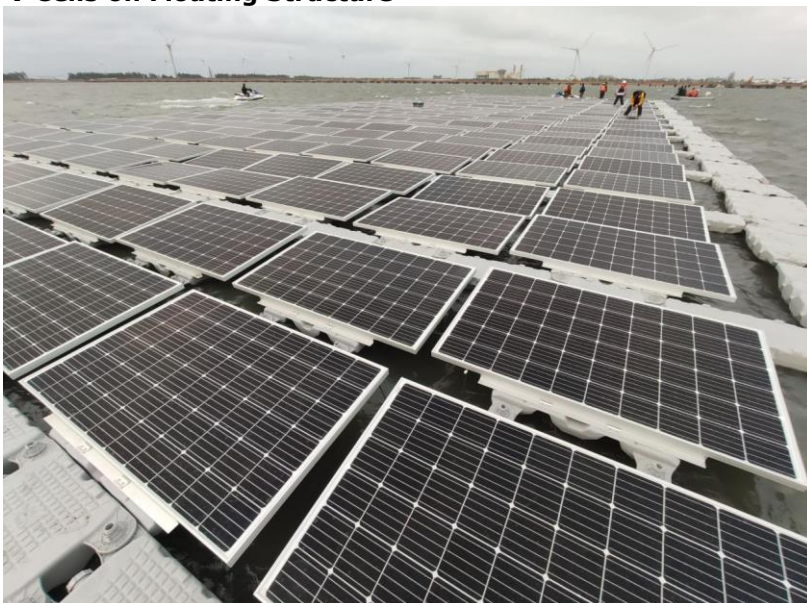
Photograph 2 – PV Cells on Floating Structure
